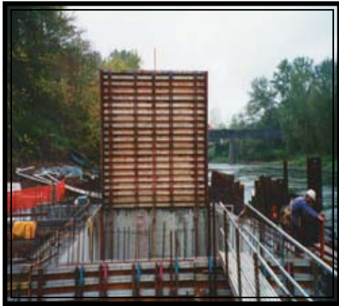
PUMP STATION - CLACKAMAS, OR
